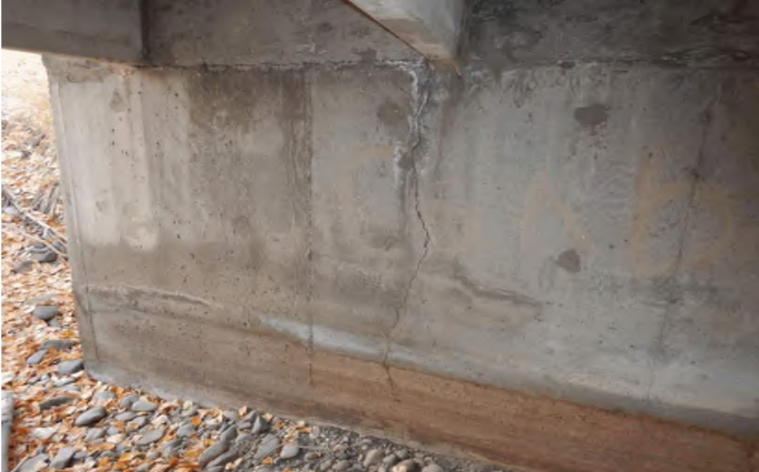
(CS3) Crack in Abutment 2 under Girder 1
