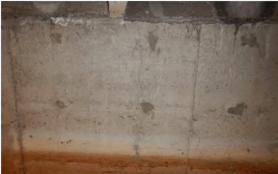
(CS3) Crack in Abutment 1 at Girder 3
