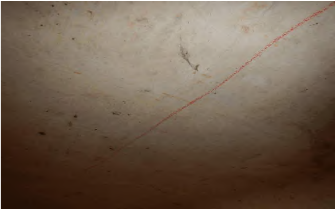
(CS3) Cracks in Top Flange of Girder 2 near Abutment 2
