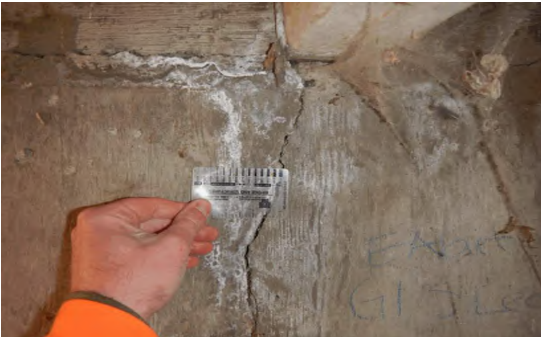
(CS3) Crack in Abutment 2 under Girder 1
