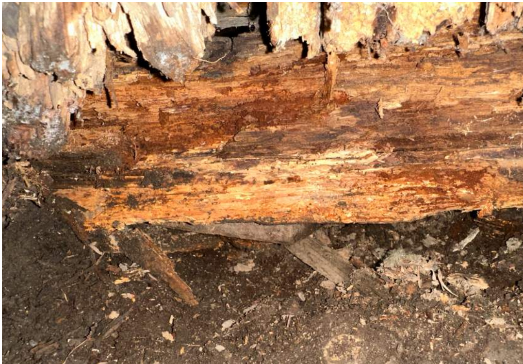
view from the hole looking up at the rotted wood
