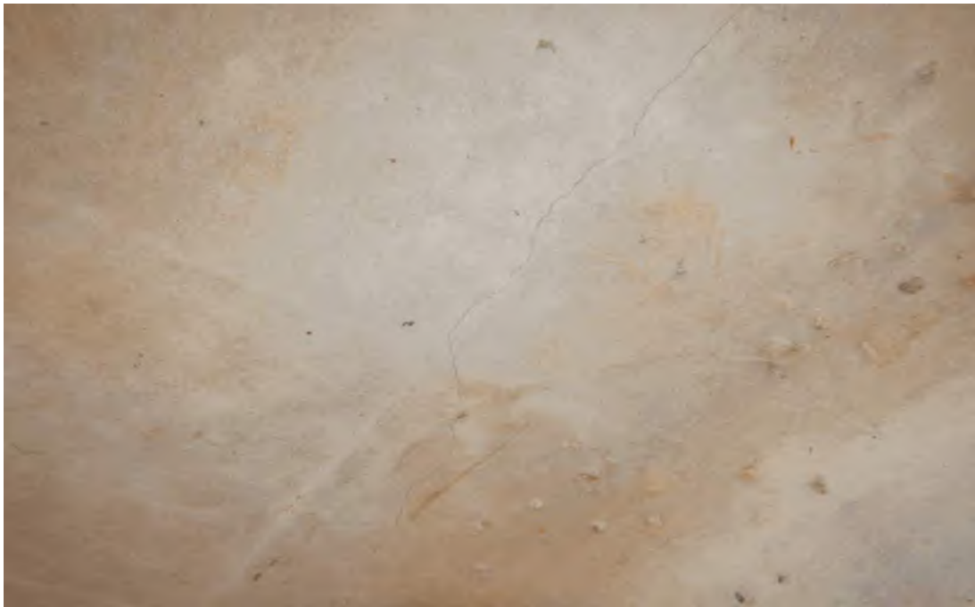
(CS3) Longitudinal Crack in Girder 4 Soffit at Abutment 1
