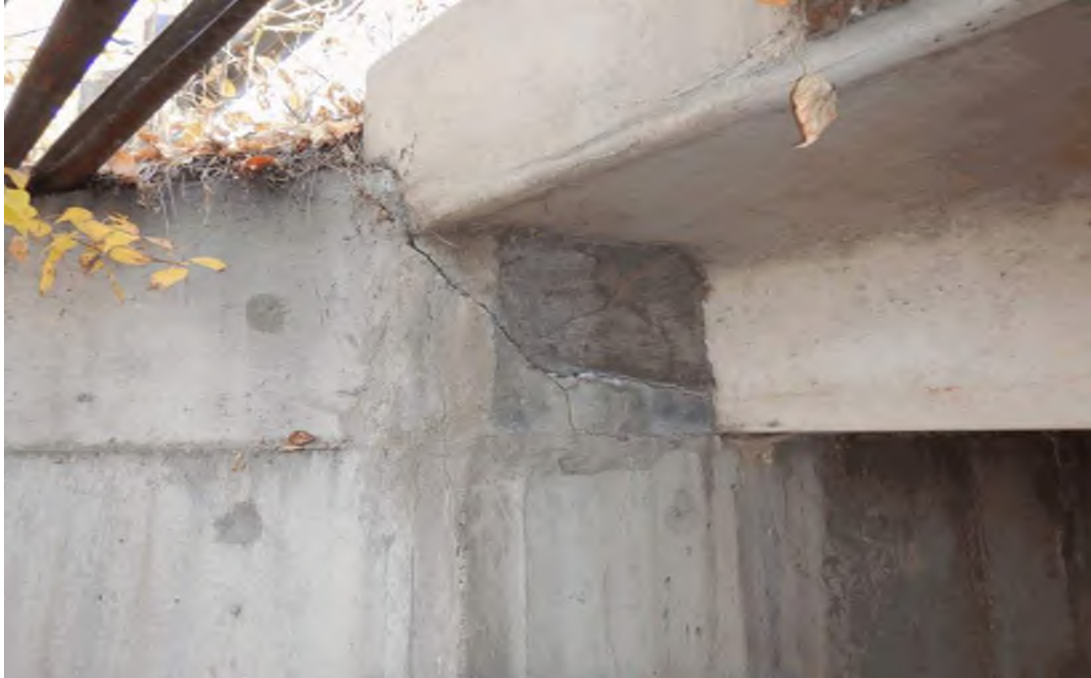
(CS3) Cracks in Northeast Wingwall
