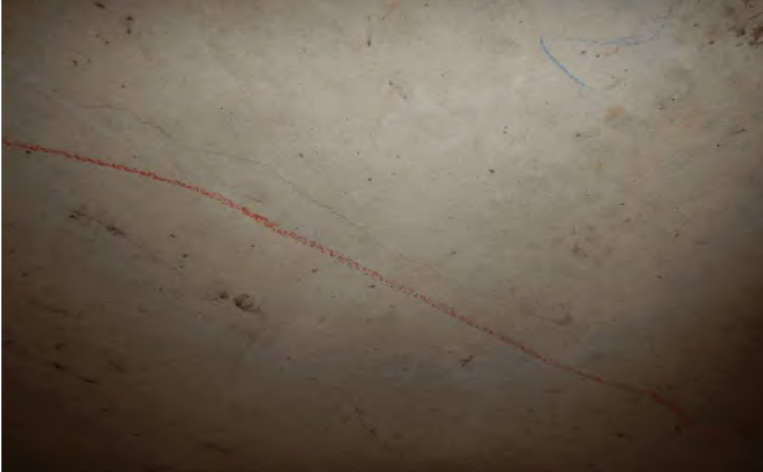
(CS3) Cracks in Top Flange of Girder 2 near Abutment 2
