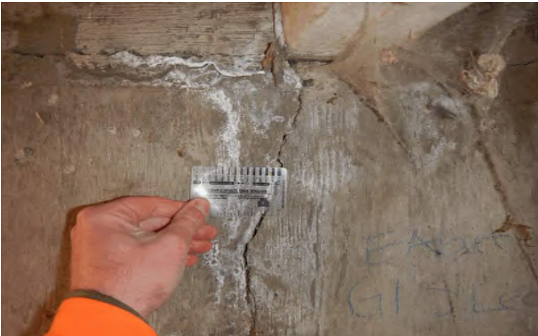
(CS3) Crack in Abutment 2 under Girder 1
