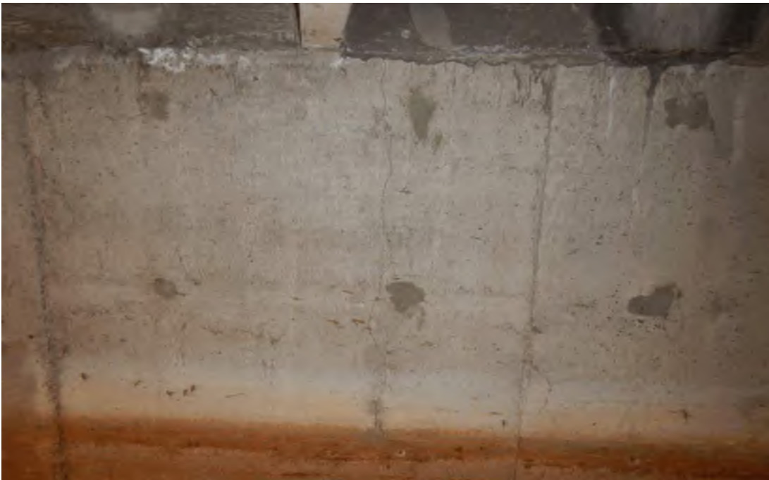
(CS3) Crack in Abutment 1 at Girder 3
