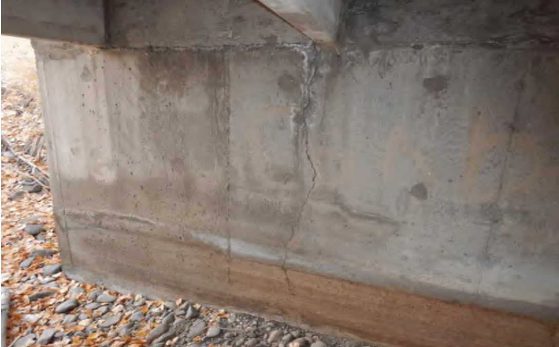
(CS3) Crack in Abutment 2 under Girder 1
