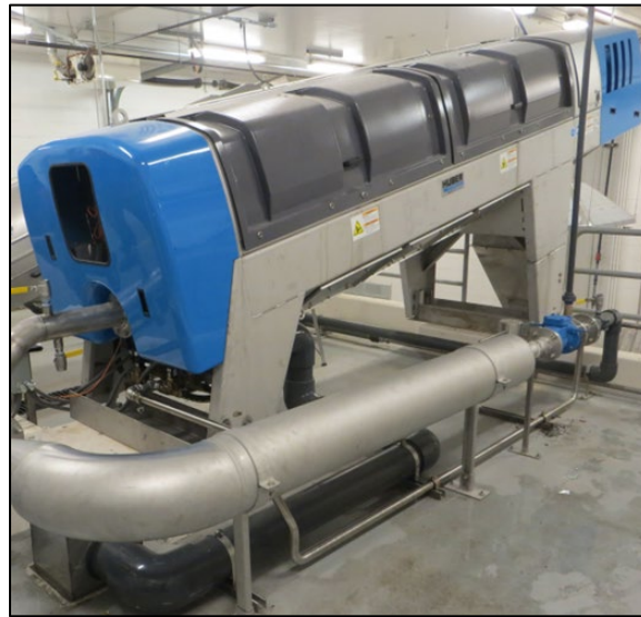
FIGURE 5-8: SCREW PRESS IN DEWATERING BUILDING
