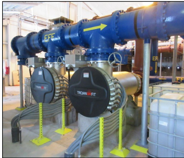
FIGURE 5-5: IN-LINE UV DISINFECTION REACTORS
